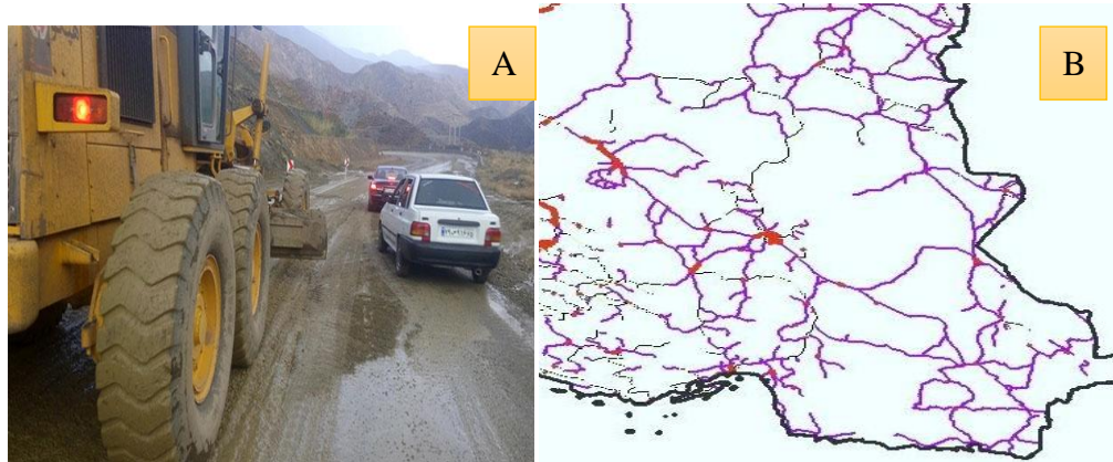
Figure 2: A) Part of the main routes in the study area, B) simultaneity of operational performance for opening the routes and utilization of the rout in the area of the study[15]
