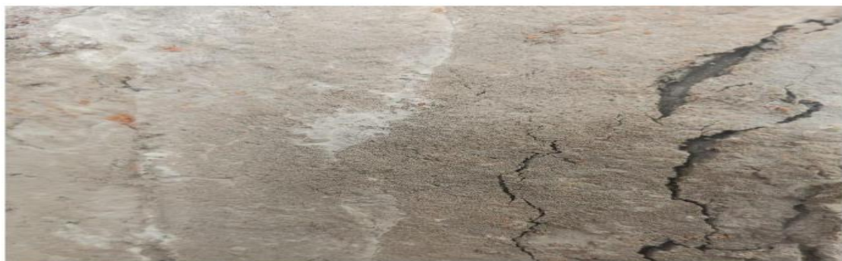
Fig. 2 - Cracks on the sides of CFRP fully wrapped beam
