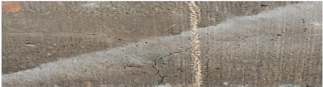
Fig. 1 - First crack on conventional beam
