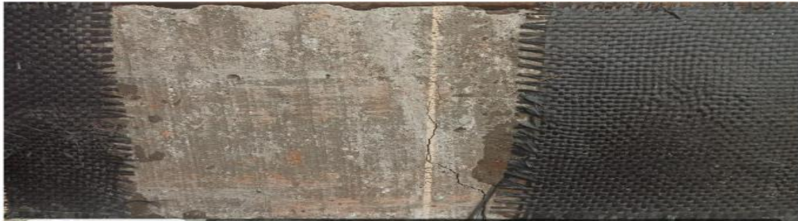
Fig. 3 - First crack on CFRP wrapped beam with 200 mm interval
