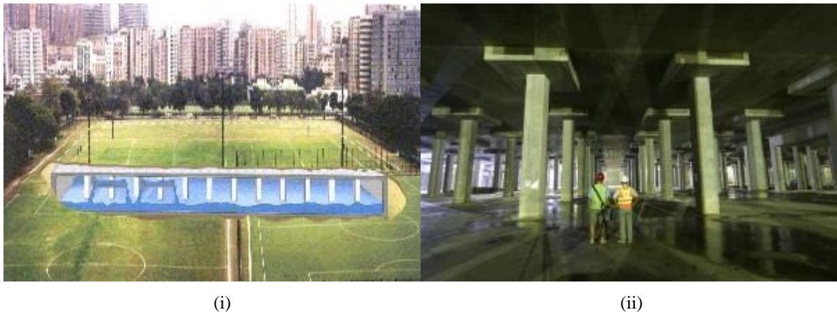
Fig. 12 - (a) Layout of Tai Hang Tung stormwater storage tank and; (b) inside view of Tai Hang Tung stormwater storage tank (DSD, 2019)
