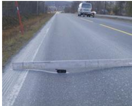
Fig. 1 Rutting phenomenon occurrence in asphalt pavement
