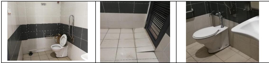
Fig. 9 - The incompliance of toilet and sanitary facilities
