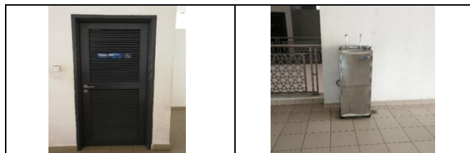
Fig. 8 - The incompliance of the device control and drinking fountain
