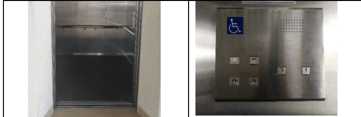
Fig. 7 - The incompliance of lift
