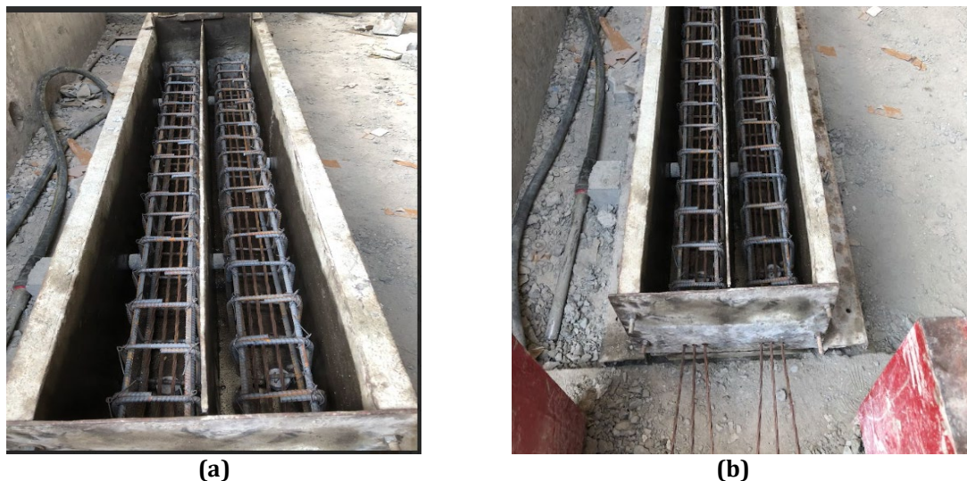
Fig. 5 Set up of reinforcement and for application of prestressing force (a) Enlarged view; (b) Zoom-out view
