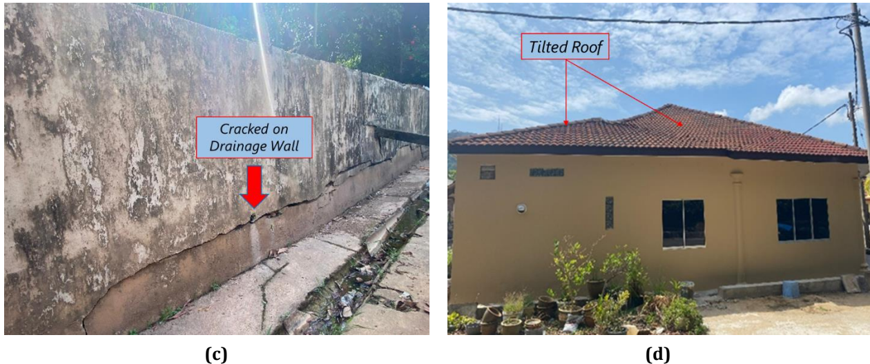
Fig. 1 Cracks observed around the Semambu residential housing area. (a) Severe cracks on a wall that have been repaired; (b) Cracks around the house porch area; (c) Cracks on the drainage wall opposite the houses; and (d) A house roof exhibiting signs of tilting
