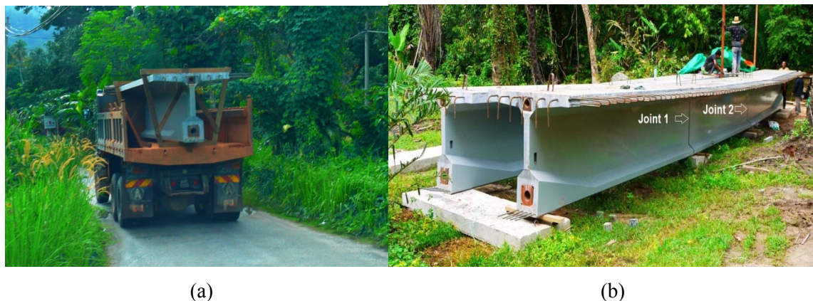
Figure 26: (a) A 10 wheels truck transporting one 6 m long UHPFRC girder segment and (b) bridge segments aligned off-site ready for post-tensioning work.
