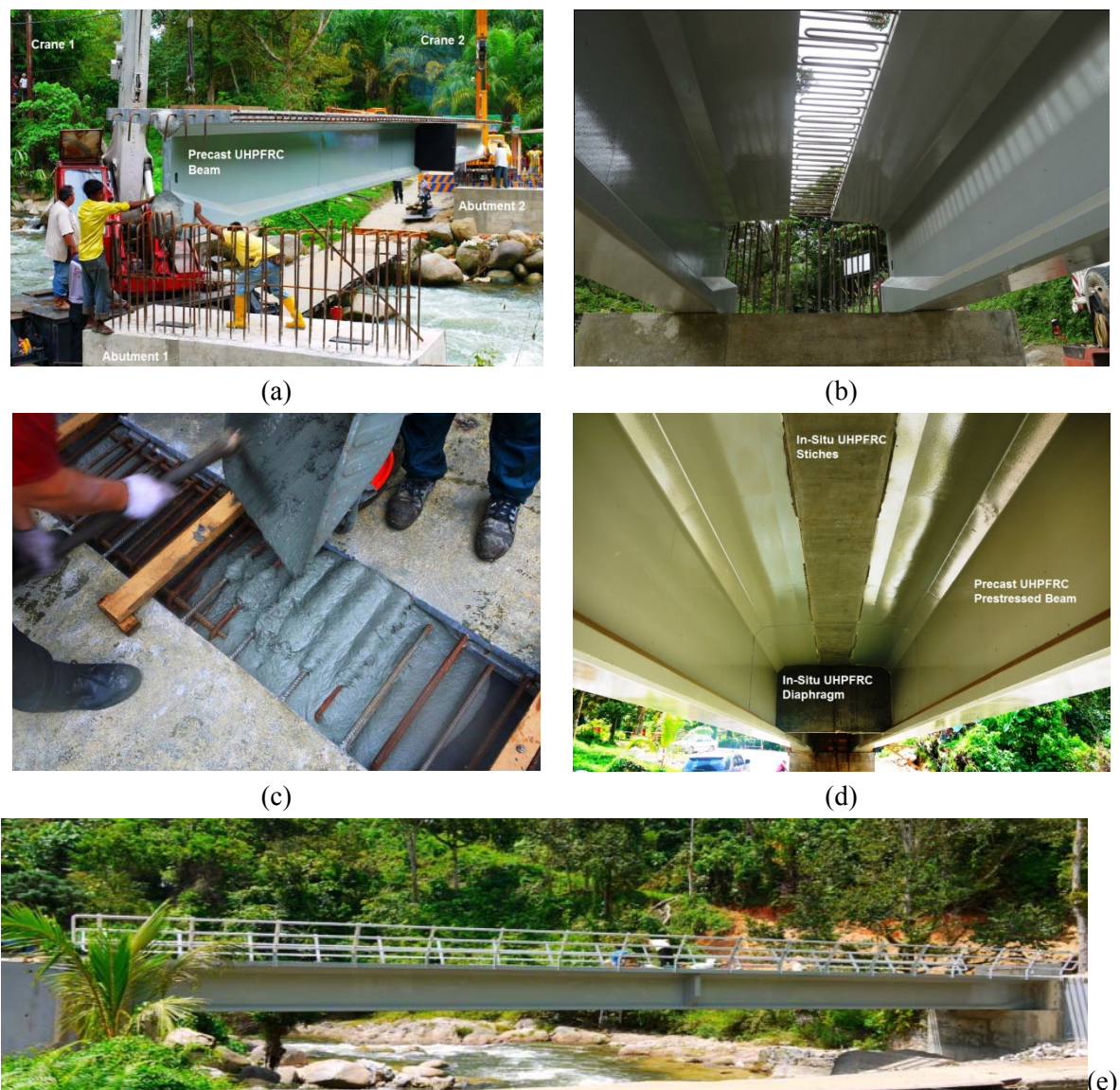
Figure 24: (a) Beams launching using two units 20 tonnes capacity mobile crane, (b) in-situ bridge joint ready for stitching, (c) placing of in-situ UHPFRC for the bridge joints, (d) view from bottom of the bridge after stitching of the bridge joint and (e) the completed Kampung Ulu Geroh Bridge.
