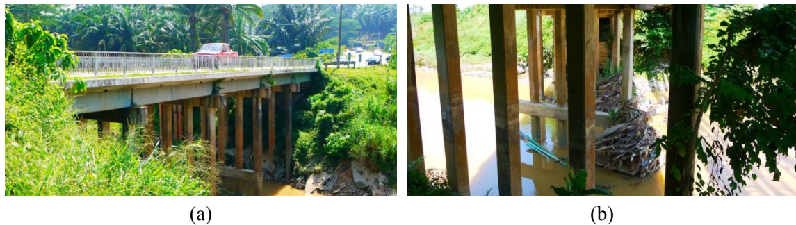
Figure 27: (a) Existing old RC bridge with four rows of RC piers at the waterway of the river and (b) debris collected at the piers.
