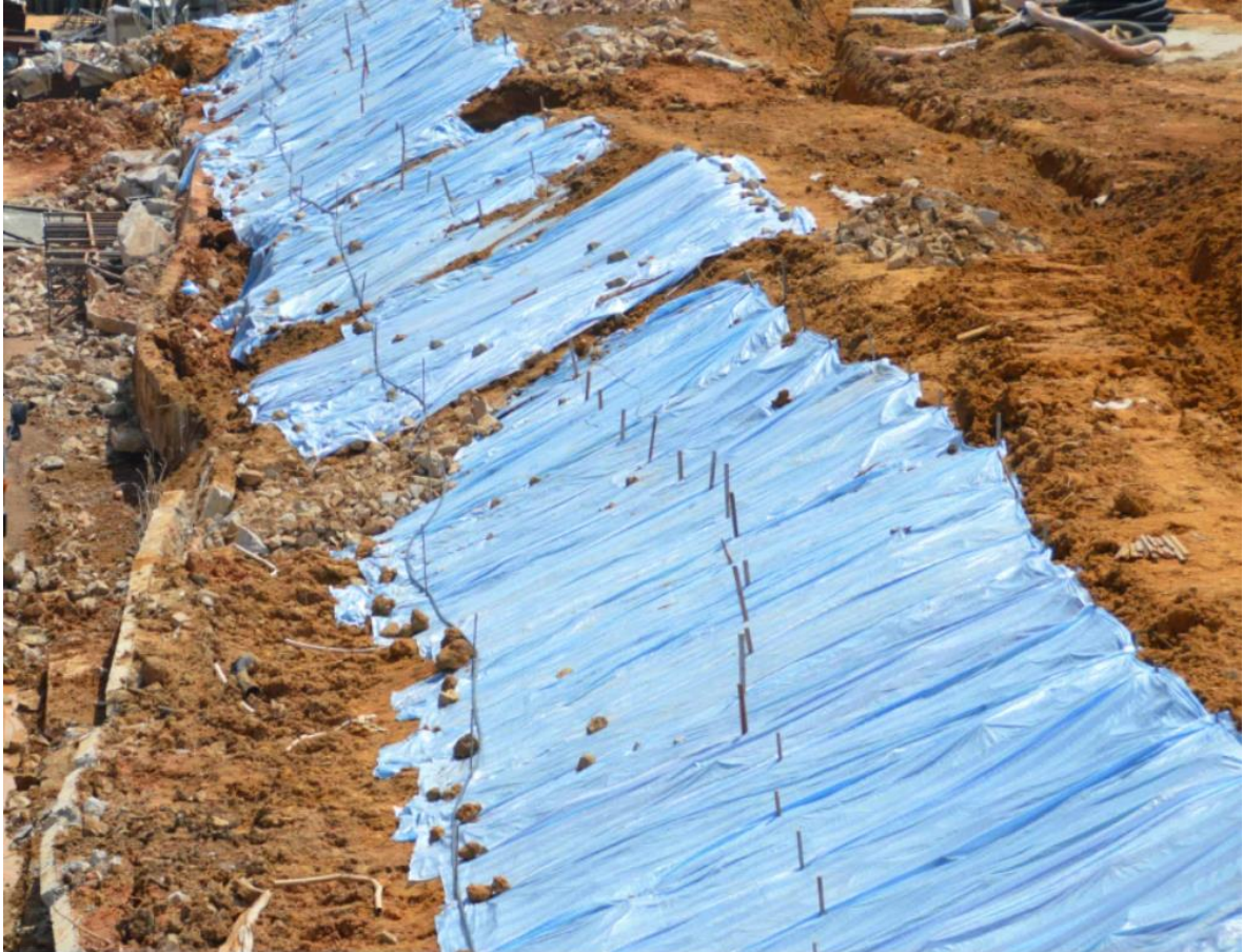
Fig. 1 (a) - 100m Long Retaining Wall Failure During Construction to be Used as Open-Ended Exercise
