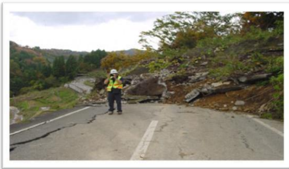
Figure 1: Situation 1- Landslide problem
