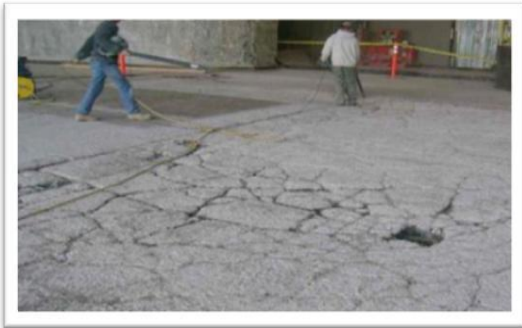
Figure 2: Situation 2- Failure of floor surface
