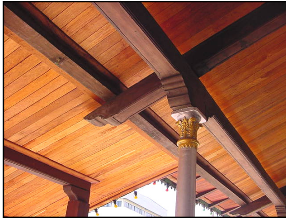
Figure 8. Post and beam construction of the lower attached roof at veranda area.
