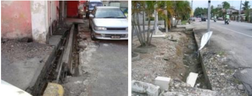
Fig. 3 - Conditions of drain in Bandar Maharani
