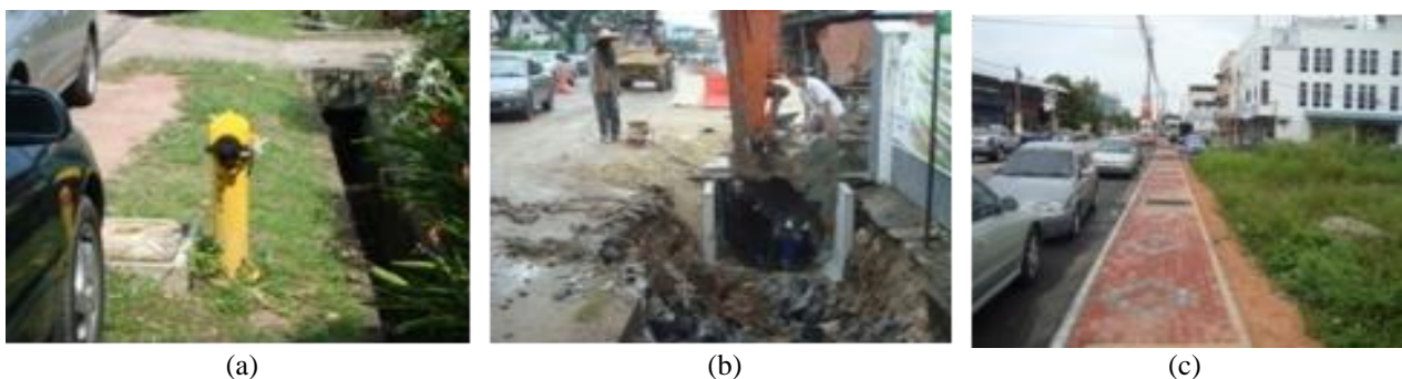
Fig. 4 - (a) Before; (b) during, and; (c) after drain upgrade works along Jalan Temenggong Ahmad (see Fig. 2)
