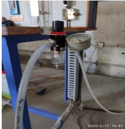
Fig. 7 - View of simple moisture filter
