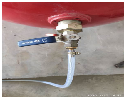
Fig. 6 - Compressor outlet valve
