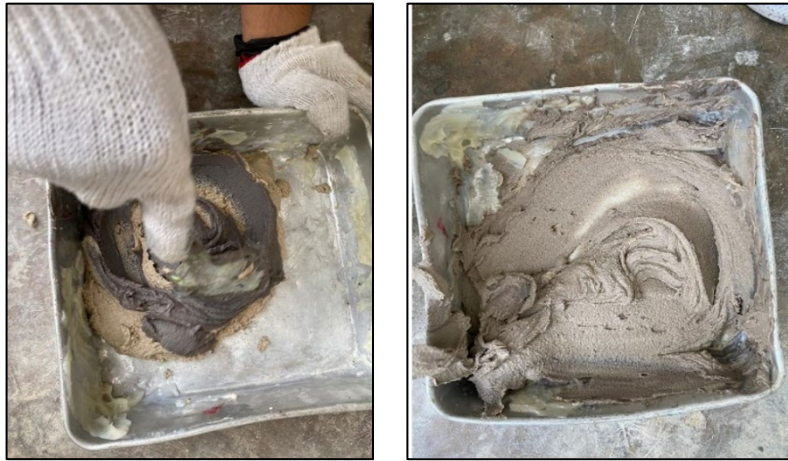
Fig. 3 The mixture of adhesive between two parts: Part A and Part B mix and concrete colour after mix
