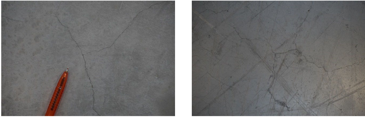
Fig. 6 Cracks were developed on the floor
