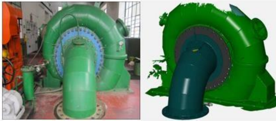
Fig. 18 - Point cloud Francis turbine complete Sancancio hydroelectric power plant 6. Runner
