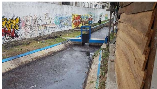
Fig. 10 - A small lock is located in the canal but is always opened
