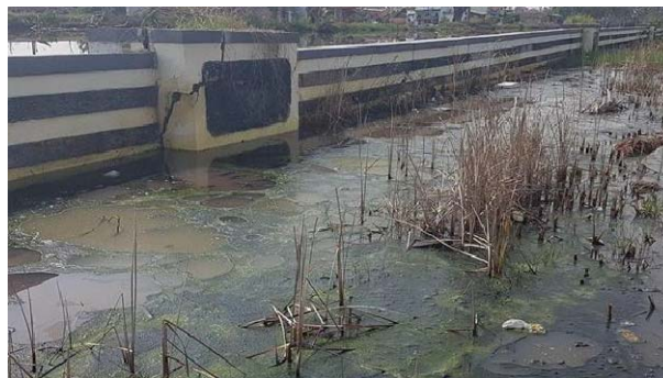
Fig. 8 - Water flows underneath and through cracks of the dike forming giant puddles
