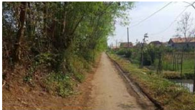
Fig. 6 - The dike alongside Sengkarang river changes from a stone-made embankment to a soil-made one
