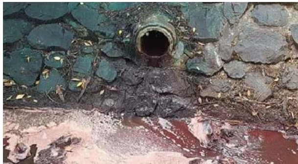
Fig. 3 - The batik industry waste water outlet into the surface water
