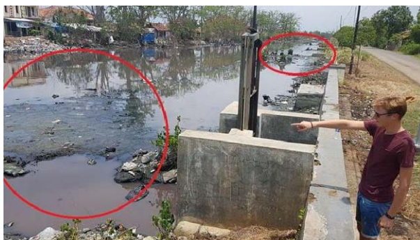
Fig. 4 - The sedimentation in the Sungai Meduri blocks a lot of the water flow
