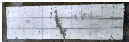
Fig. 18 - Crack happens on beam samples for the first attempt
