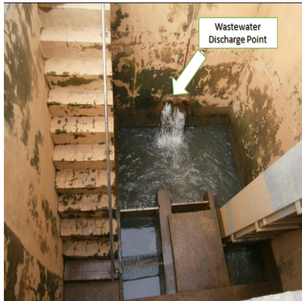
Fig. 2 - Institutional wastewater discharge point, sewage plant, UTHM
