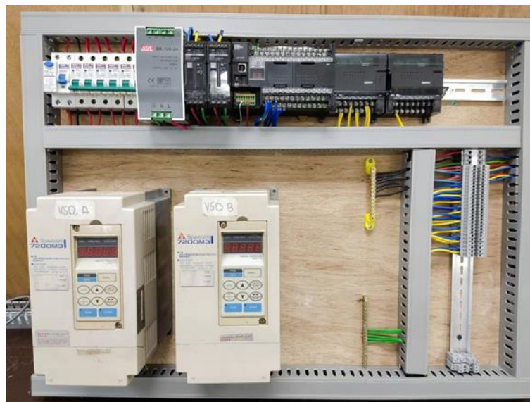
Fig. 3 - (a) PLC Panel
