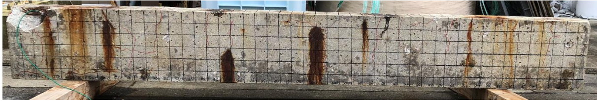
Fig. 6 - Defective appearances of the RC beam
