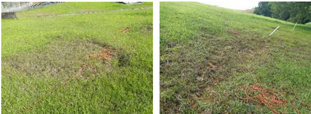
Fig. 2 - Water seepage occurred at #Berm 5
