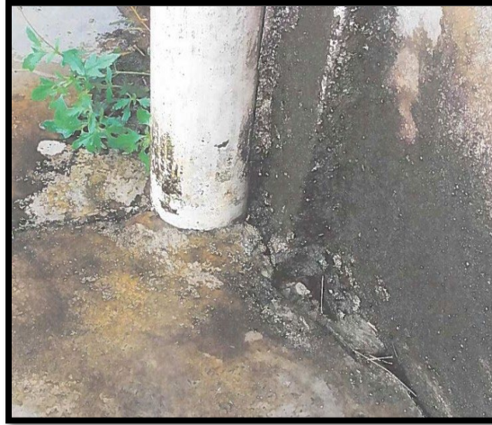
Fig. 1 Rotting wall and column
