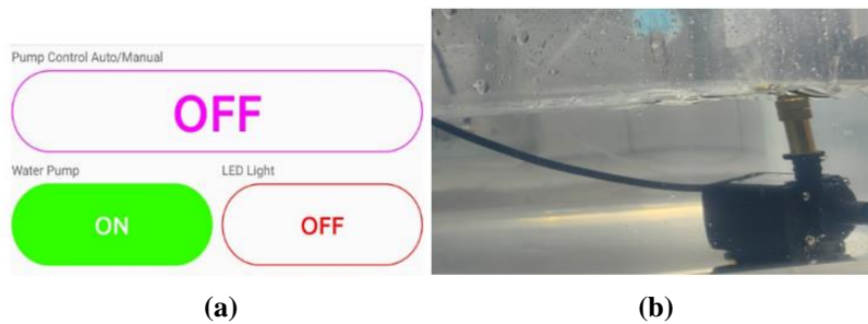
Fig. 14 Water pump control unit view (a) Blynk view; (b) Real view
