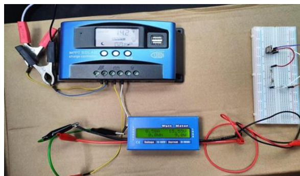
Fig. 17 Overcurrent protection testing circuit
