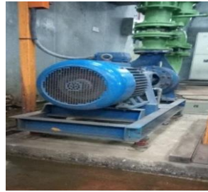
Figure 4: Motor for chilled water pump 4
