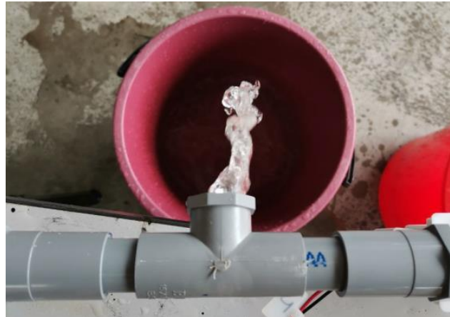
Figure 9: Leakage in section 1
