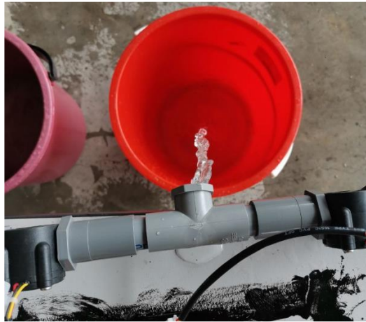
Figure 12: Leakage in section 2
