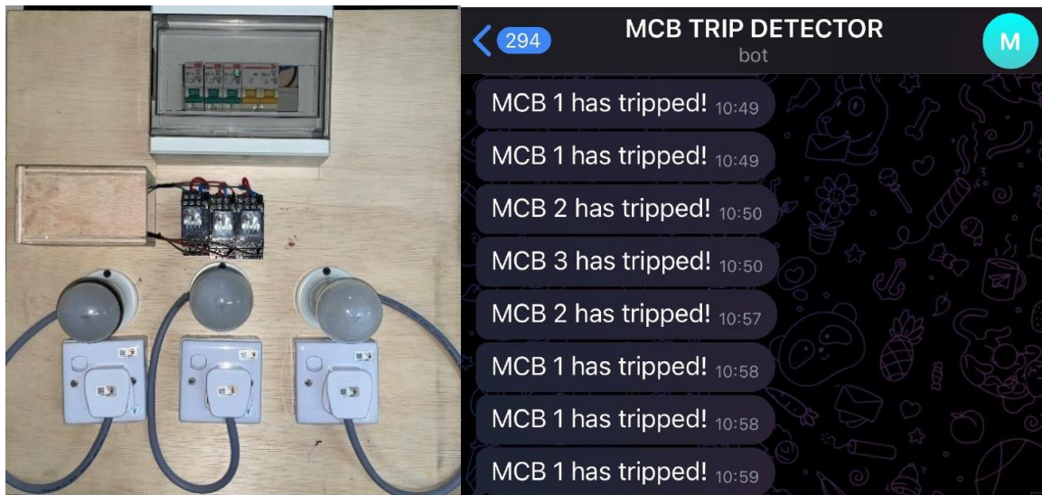
Fig. 3 (a) Prototype of the Miniature Circuit Breaker Trip Detector, (b) Notification from Telegram Bot
