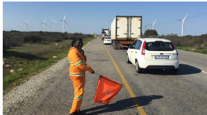
Figure 1: Flagman working in high risk hazard condition
