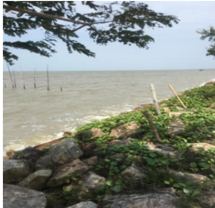
Figure 1: The condition of SCE during high tide
