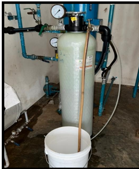
Figure 3 : Softener equipment for treating hard water
