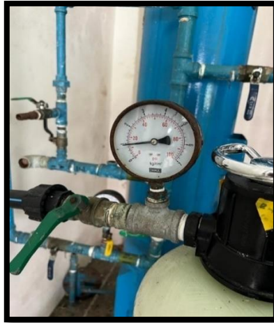
Figure 2 : Manual hand valve, pressure gauge and softener handle
