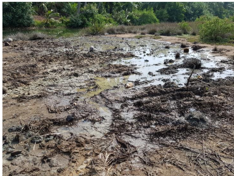
Figure 2: Close-up of the seepage happened at the inland area
