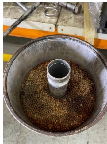
Figure 14: Desiccant gel that has been used 2 years inside the air dryer
