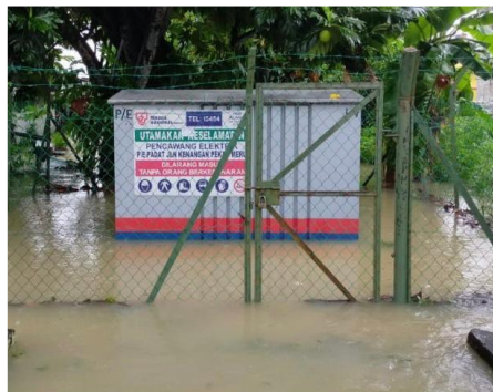
Figure 2: Unmanned substation got flooded at Meru, Selangor .
