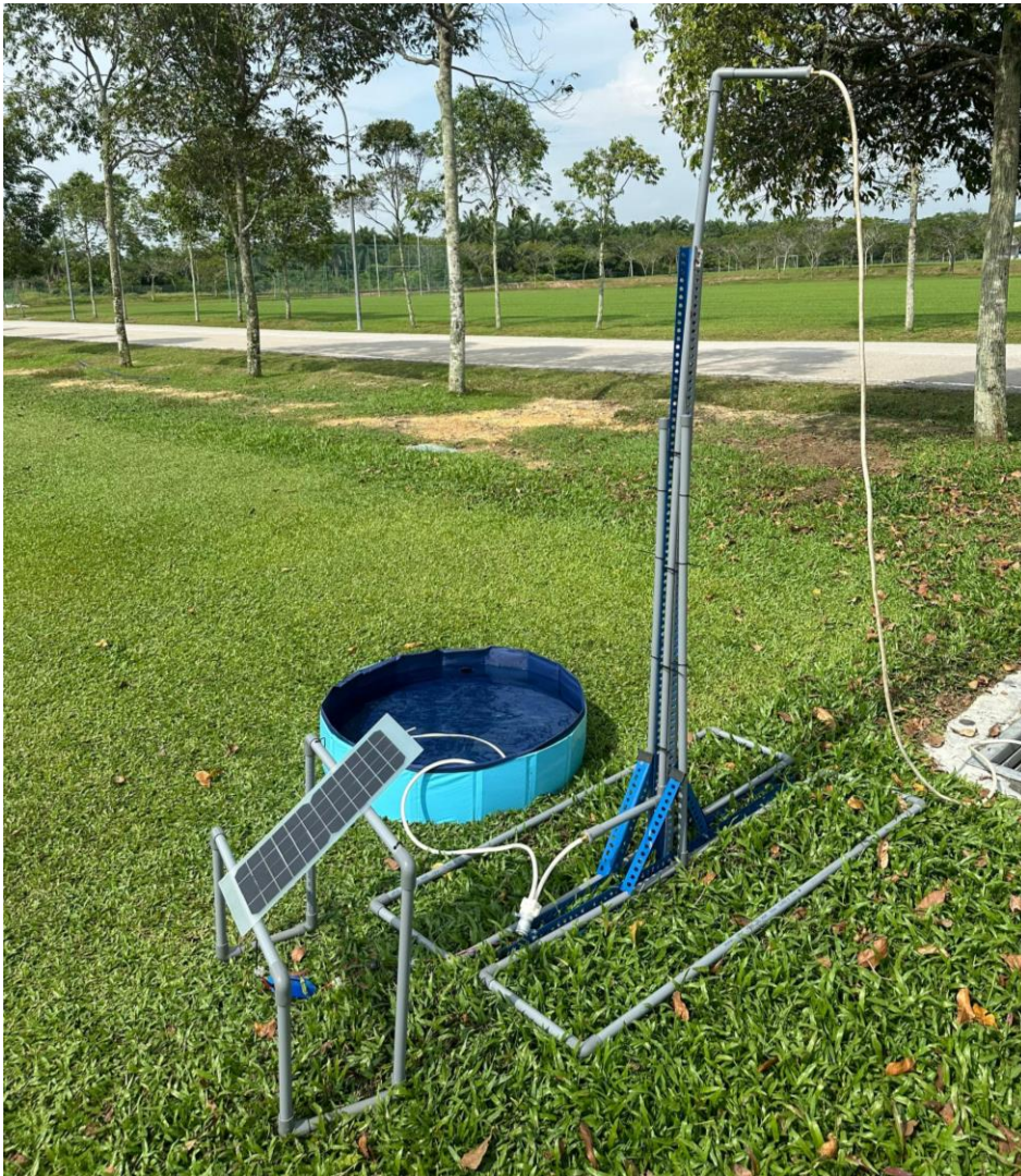
Fig. 5 The Actual Setup of The Off-Grid Solar System Without Using Battery Storage
