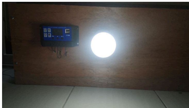
Figure 7: the working PV power system
