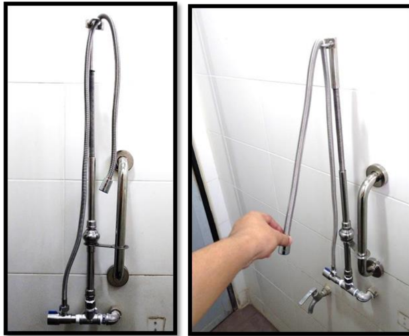
Figure 5: the stainless-steel water hose pipe using with flexible spring has been completed
