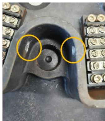
Figure 4: Defect on junction box housing due to shaft's bolt
