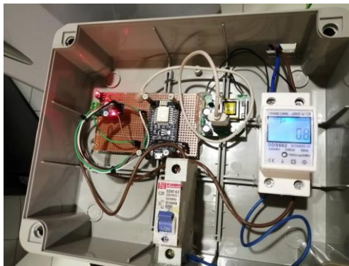
Figure 5: Results shown in Energy Monitor IEC62053-21
