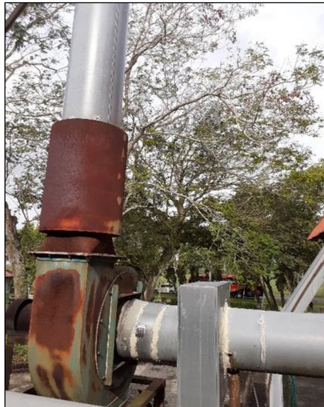
Figure 5: Condition of exhaust stack due to oxidation process
