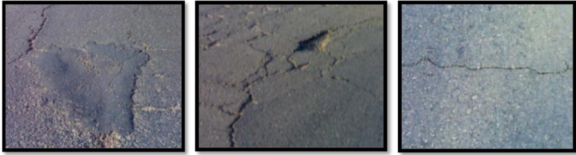
Figure 3.1: The surface defects that occurred along the road networks.
