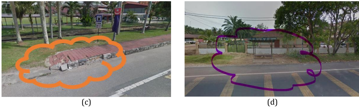
Fig. 2 Examples of recurring safety issues; (a) poor sign at SK02; (b) uneven road surface at SK02; (c) damaged footpath at SK10; (d) no provision of bus lay-by at SK03
